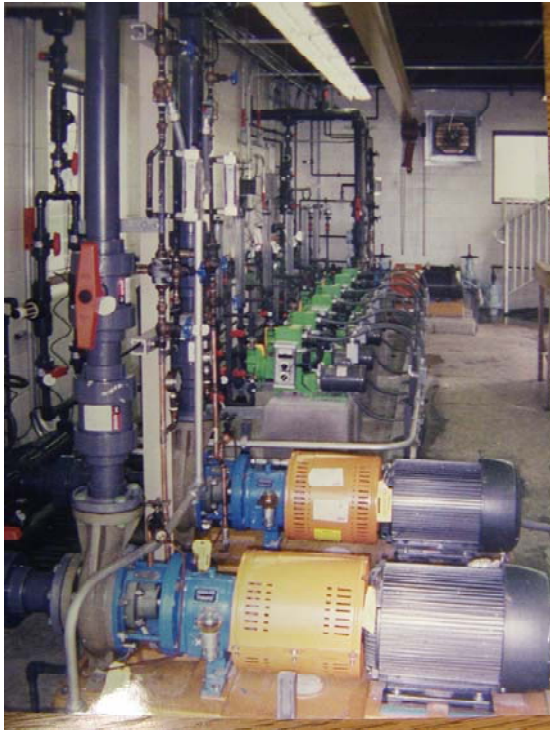
Picture B: Back River WWTP, City of Baltimore, Maryland (36,000 CFM)
