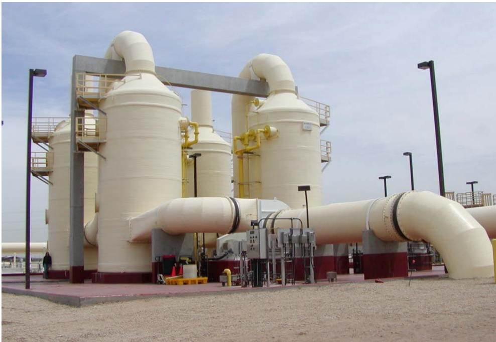
Picture #2: City of Phoenix 91st Avenue WWTP, Arizona (120,000 CFM)
