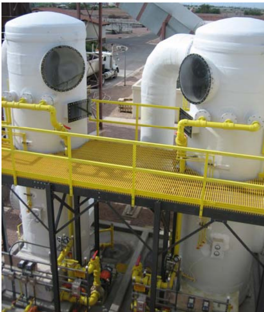
Ocotillo Water Reclamation Plant, Chandler, AZ (11,200 CFM)
