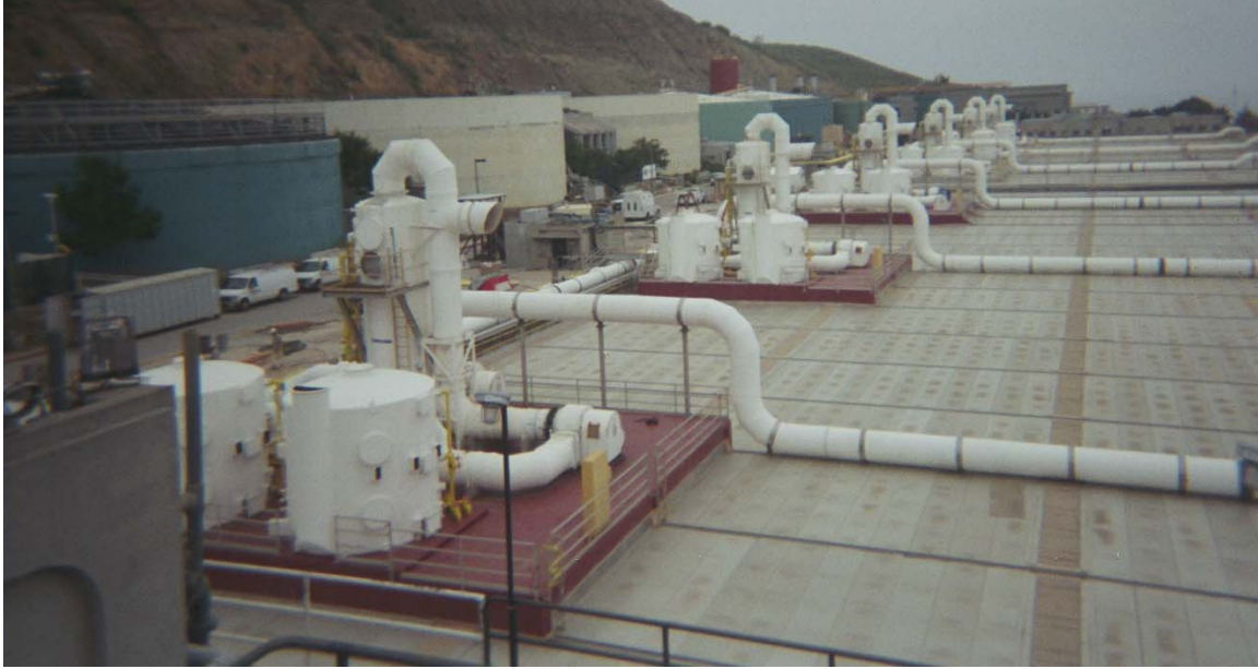
Pt. Loma WWTP Scum Removal, Accelerated Odor Control and Concrete Restoration, Pt. Loma, California (132,000 CFM)
