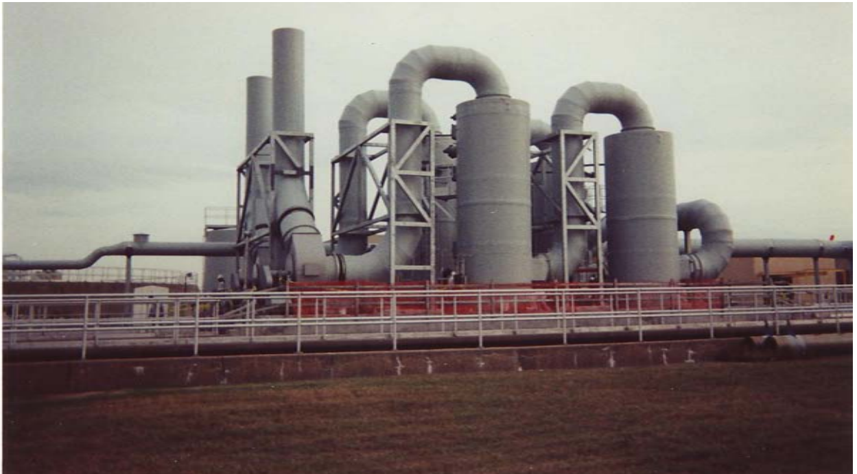
Picture #A: Army Base Wastewater Treatment Plant, Norfolk, Virginia (58,000 CFM)
