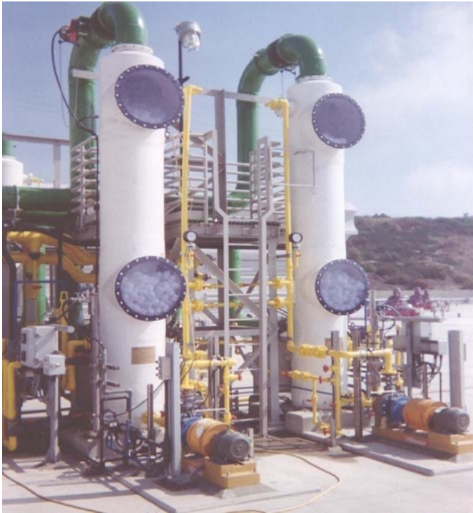
Hyperion Treatment Plant, Los Angeles, California (6 systems totaling 32,000 CFM)
