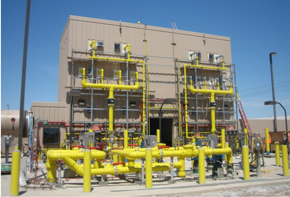
Picture #1: UP01 91st Avenue WWTP, Arizona (75,000 CFM)
